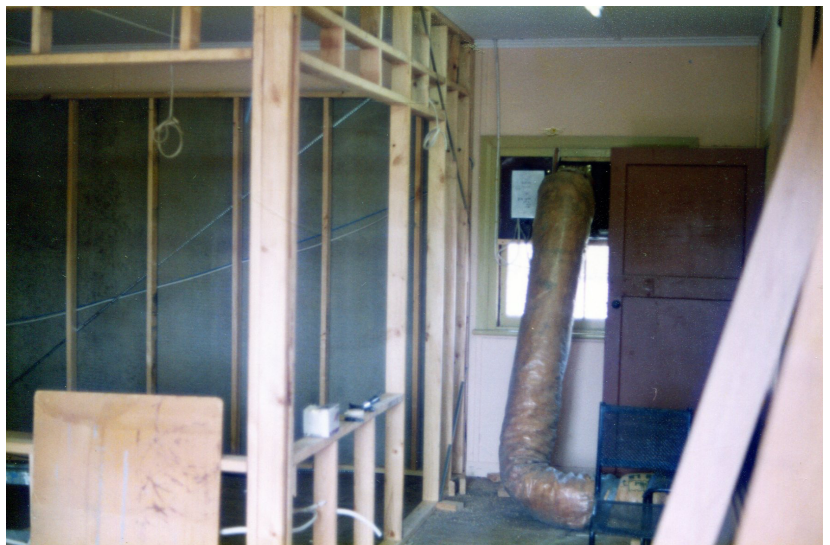
Early days of construction of SWR's studio at the Blacktown Showgrounds, which would variously remain in service through a few upgrades right up to 2022.
