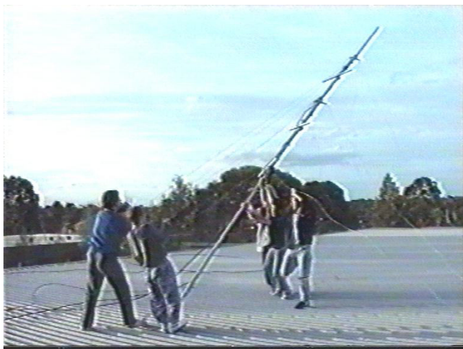
Above : The antenna is raised atop the roof of the Poppondetta Road Emerton site.
