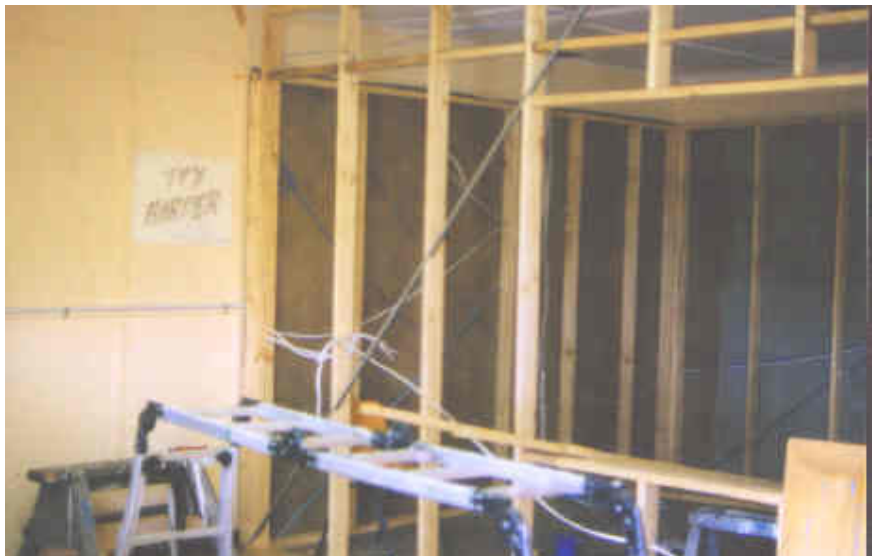
Photo of the very first days of occupation of the Blacktown Showgrounds site in mid 1999, showing construction of studio one proceeding at a blistering pace towards opening a mere two weeks later.
