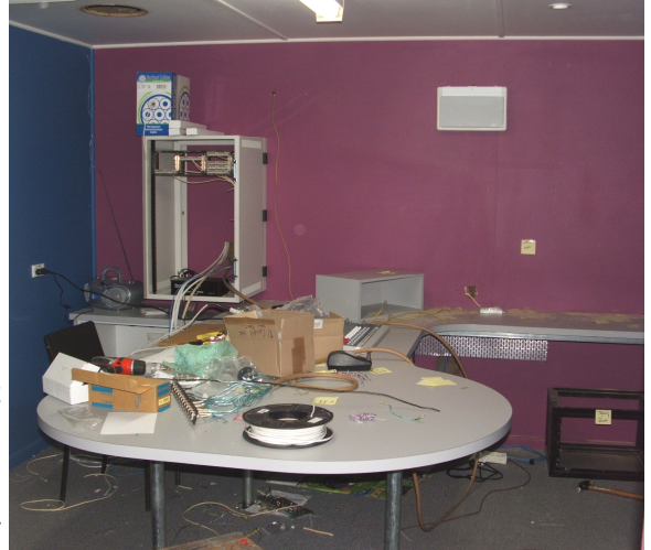
Construction of the 2006 Studio Rebuild commences. This robust design would see the station successfully through the next 17 years of service.
