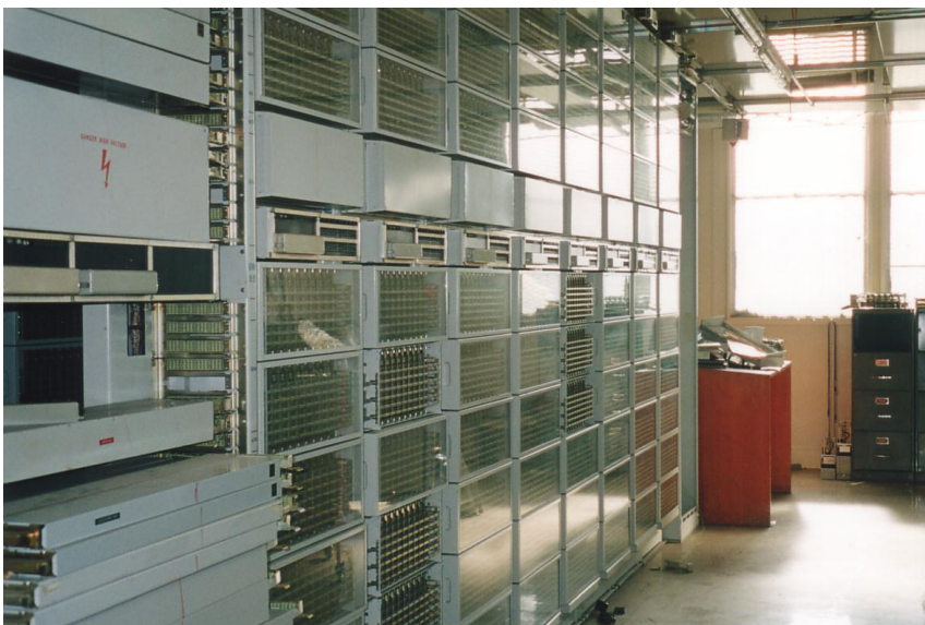
Above : Typical “Crossbar” telephone exchange equipment, as found in all Western Sydney exchanges in the 1990s.
