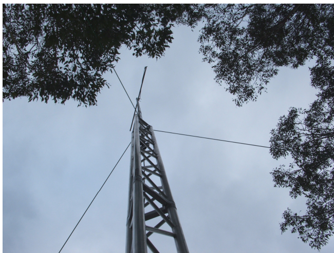
Australia Day 2009—A manually erected 9m Tri Truss tower supports an FM link antenna
